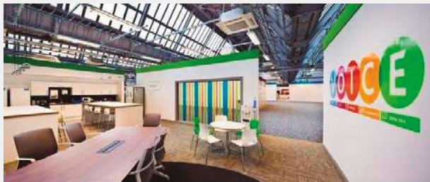
CAPITA call centre. UK. 11 ECO G 3-Pipe units. Over 150 indoor units in meeting rooms and open-plan areas. Intelligent touch screen controller, the CZ-256ESMC2.
